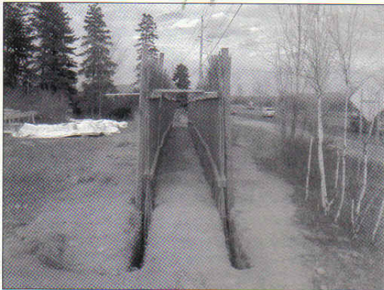
Figure 2. Stems are assembled tightly in a wooden frame and installed upright in two trenches set 1.2 m (4 ft) apart.
